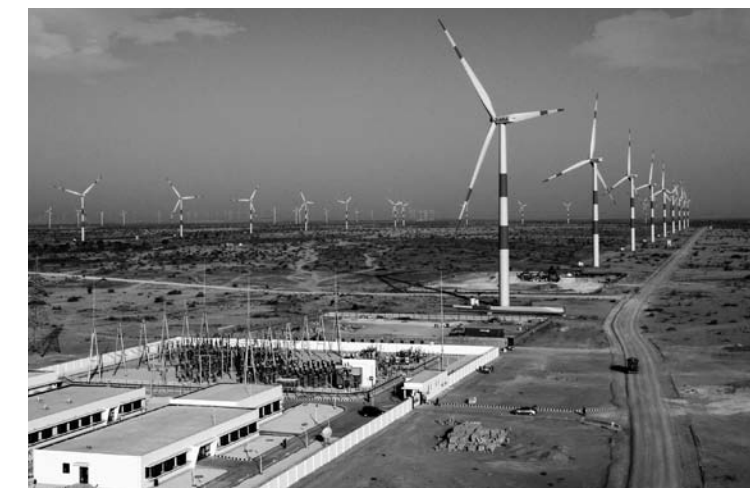
Hawa operations facility and wind turbines
