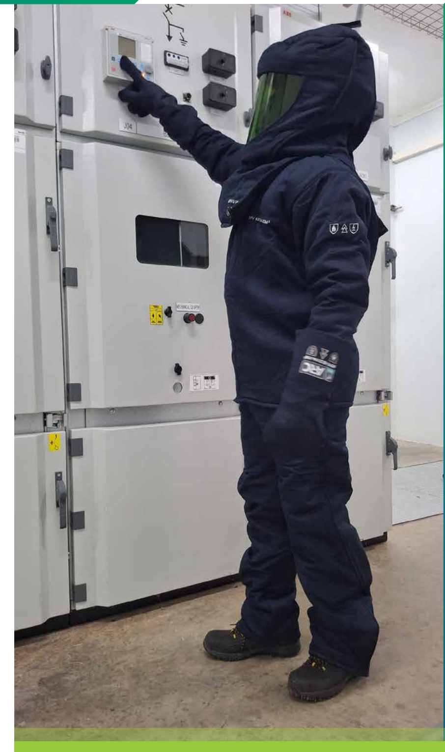
Golomoti employee working in the 22kV switching room, wearing arc flash protective gear.
